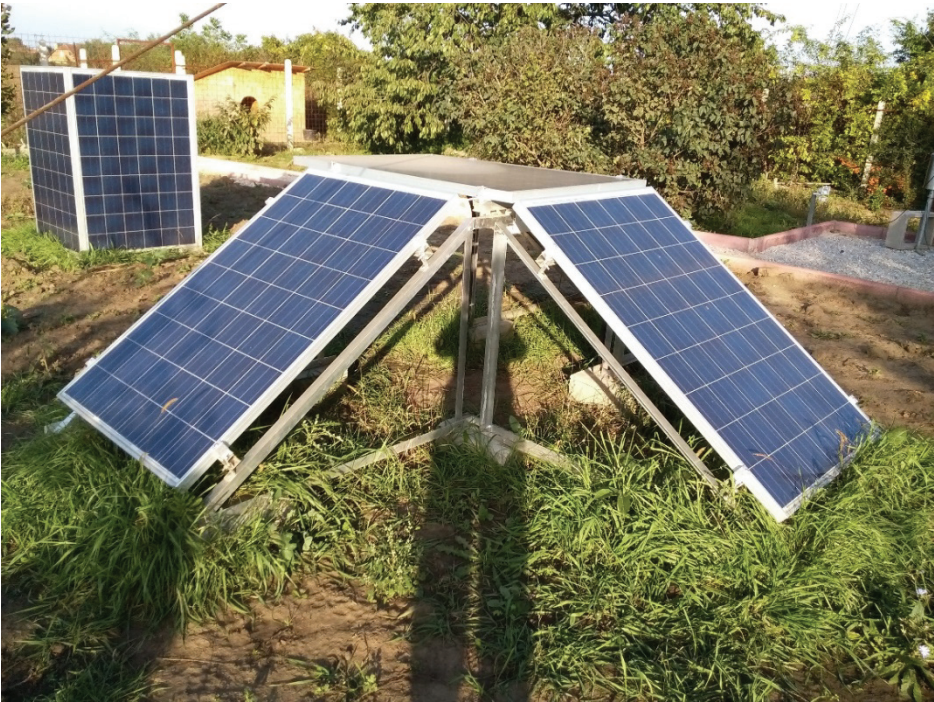
Fig. 2. The PV arrays at the station.
